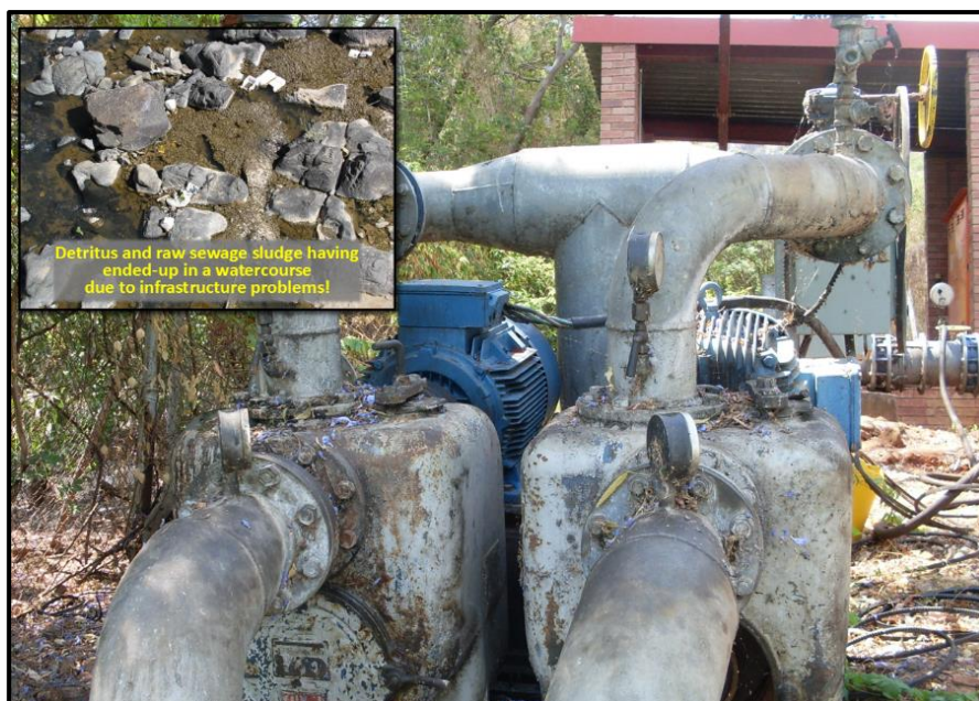
FIGURE 2: Vandalism, ageing infrastructure and insufficient maintenance of sewage infrastructure cause water pollution, which contributes to eutrophic conditions in receiving water resources. Main photo: © P. Venter; Insert photo: © J.J. van Wyk.
