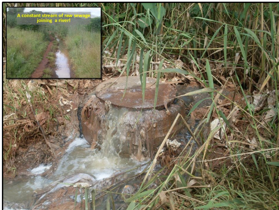
FIGURE 1: Streams of poorly treated and untreated sewage and industrial wastewater, exacerbating the effects of anthropogenic eutrophication, have become an all too familiar face in many parts of the country. Photos: © P. Venter.
